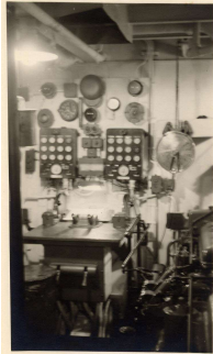
Engine room control panel
